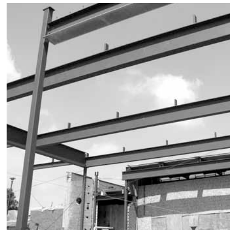
Construction progress, and an overview of the work, can be viewed at www.hclib.org , under "Northeast Library."
